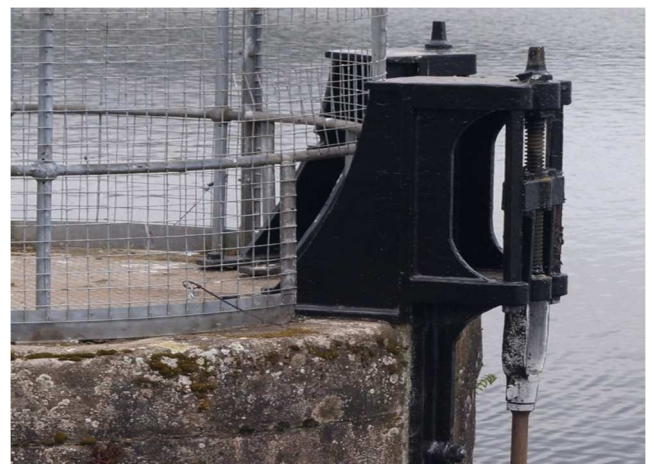
Figure 99. Gartmorn dam slide valves.
