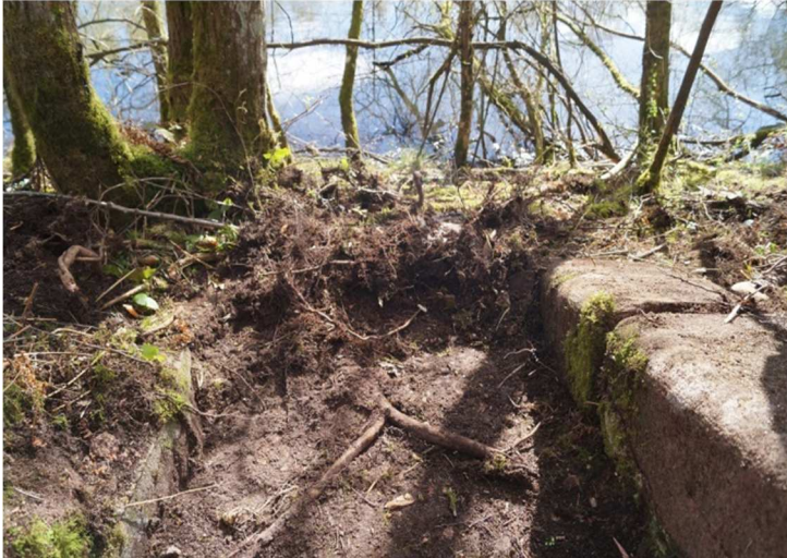
Figure 121. Inlet three spillway into pond.
