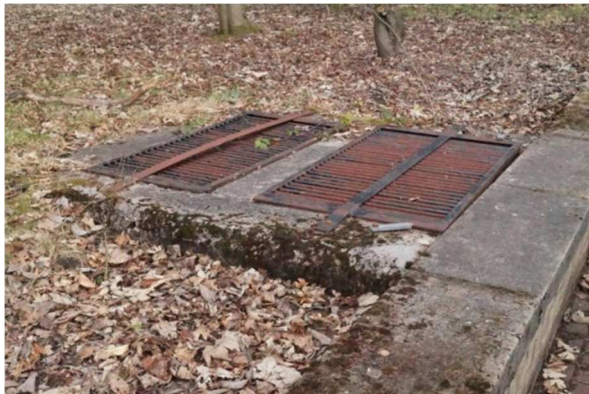
Figure 109. Filter bed weir top.
