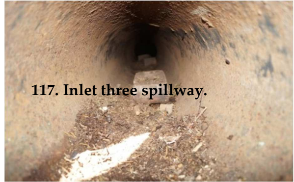
Figure 120. Pipe at inlet three.
