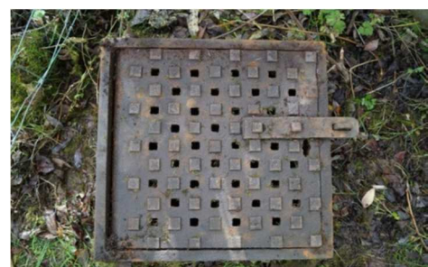
Figure 72. Cast iron cover.
