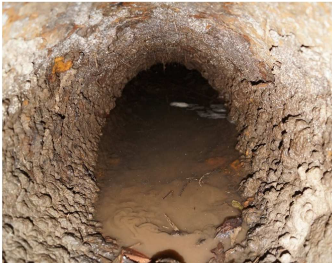
Figure 69. Iron pipe looking downstream.
