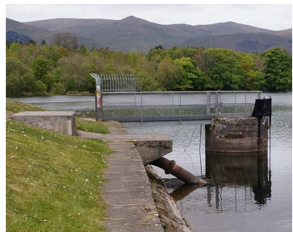
Figure 115. Pipeline at water tower.
