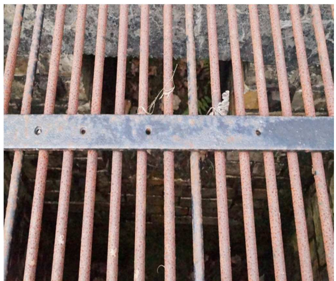
Figure 110. Filter bed weir top.
